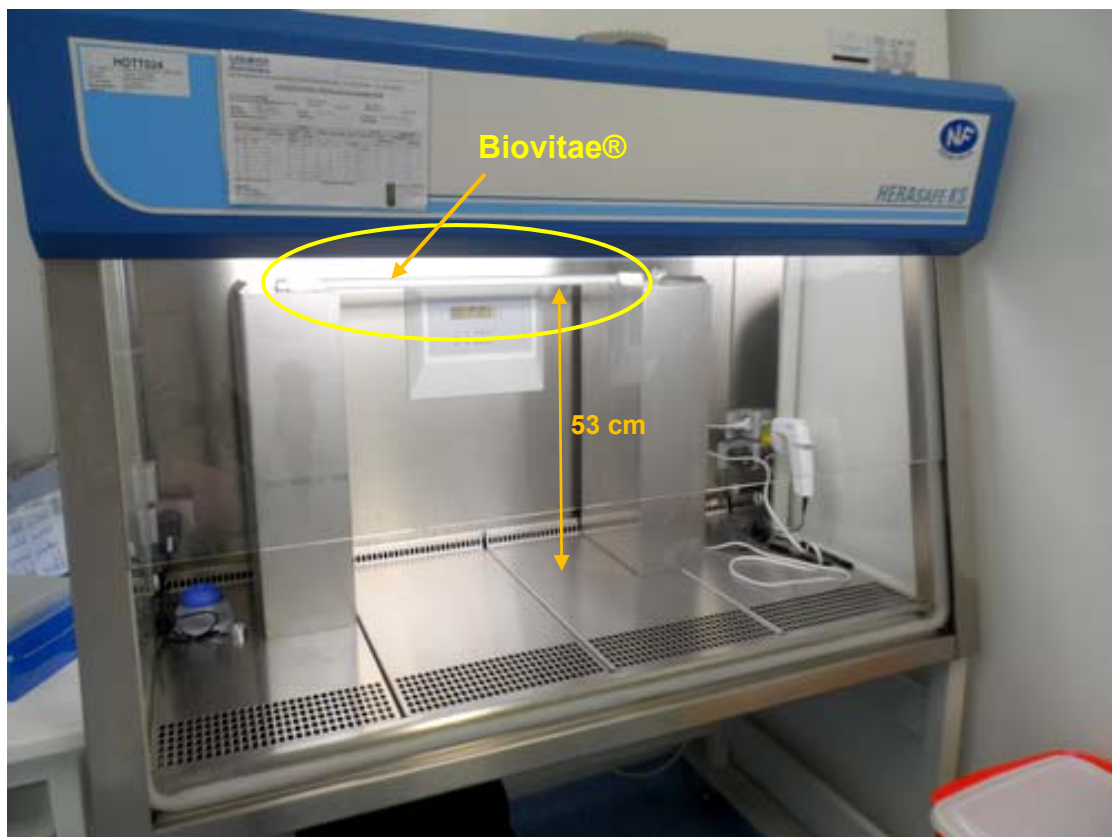
Fig 2: Biovitae® lamp installed in a BSC II of the BSL3 laboratory with a height of 53 cm from the work surface.
